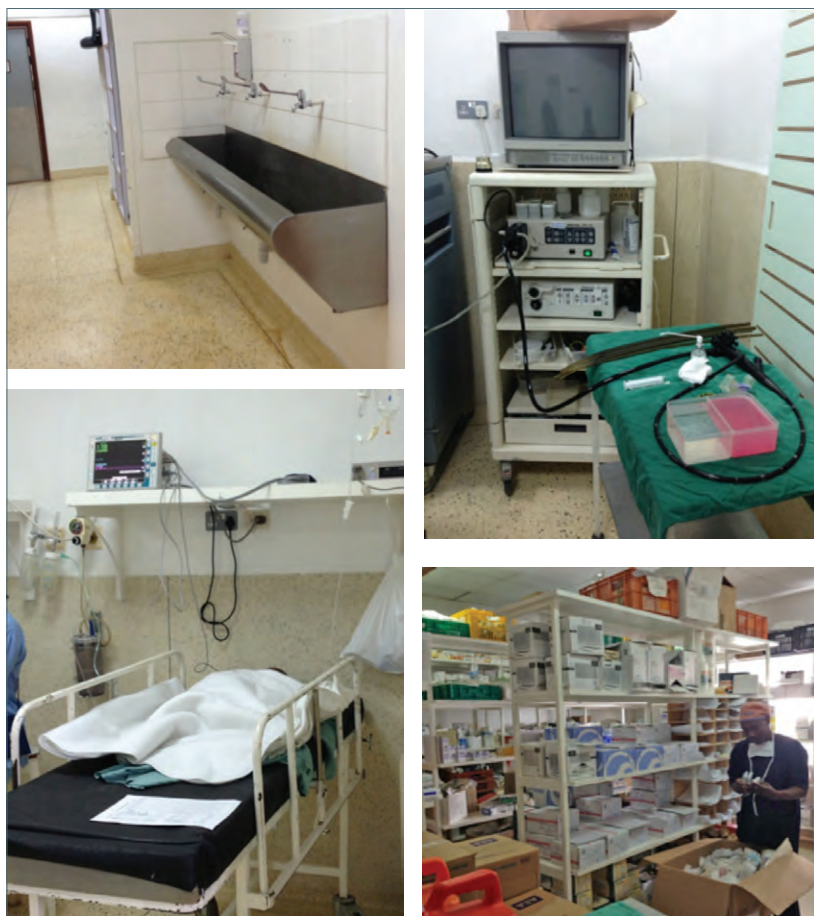
Exhibit 9: Surgical Facilities at AIC Kijabe Hospital Clockwise from top left: hand wash sinks outside operating theater; endoscopy/minor procedure suite; operating theater mini-store room with attendant; post-operative recovery area with wall oxygen, suction, and vital sign monitoring. Source: Case writers.
